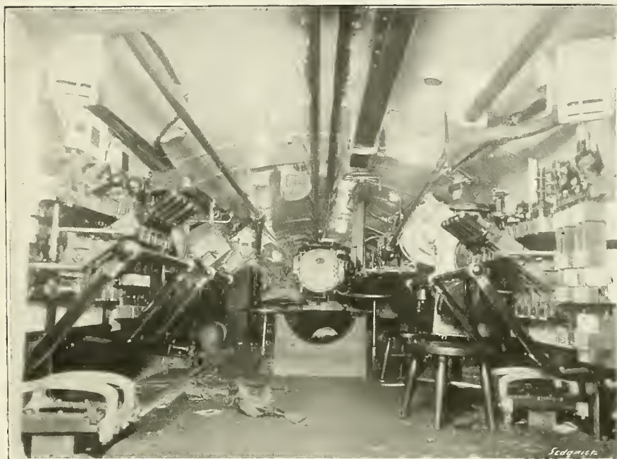
SUBMARINE INTERIOR, VIEW IN MOTOR CONTROL ROOM.
