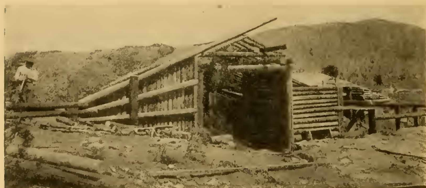
FIG. 111.—Exterior view of a large potato storage cellar in process of construction on the Sweet ranch, Carbondale, Colorado, showing construction of vestibule entrance and the covering of roof with straw.
