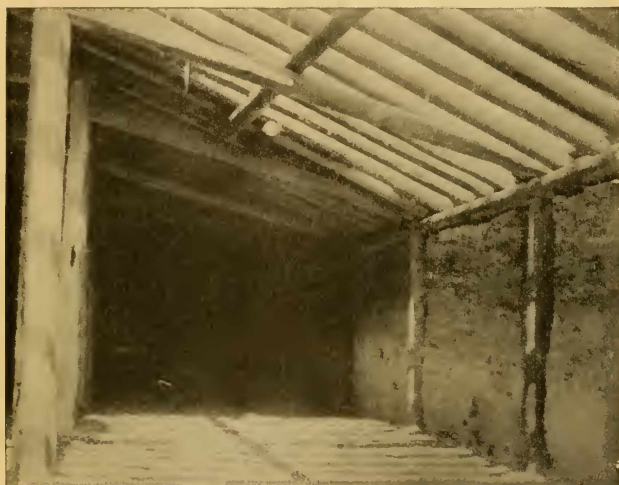
FIG. 121.—View showing earthen wall with plate supporting posts recessed into the bank. On the Sweet ranch, Carbondale, Col.
