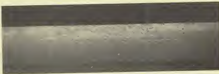
FIG. 19. CLIP REMOVED REVEALING BADLY CORRODED AREA BENEATH
