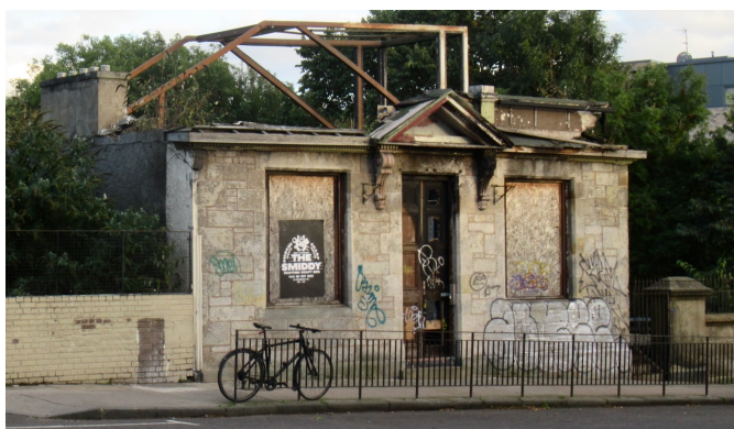
Derelict Bonnington Bridge Bar
