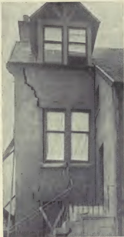
Houses cracked by underground workings, Motherwell
