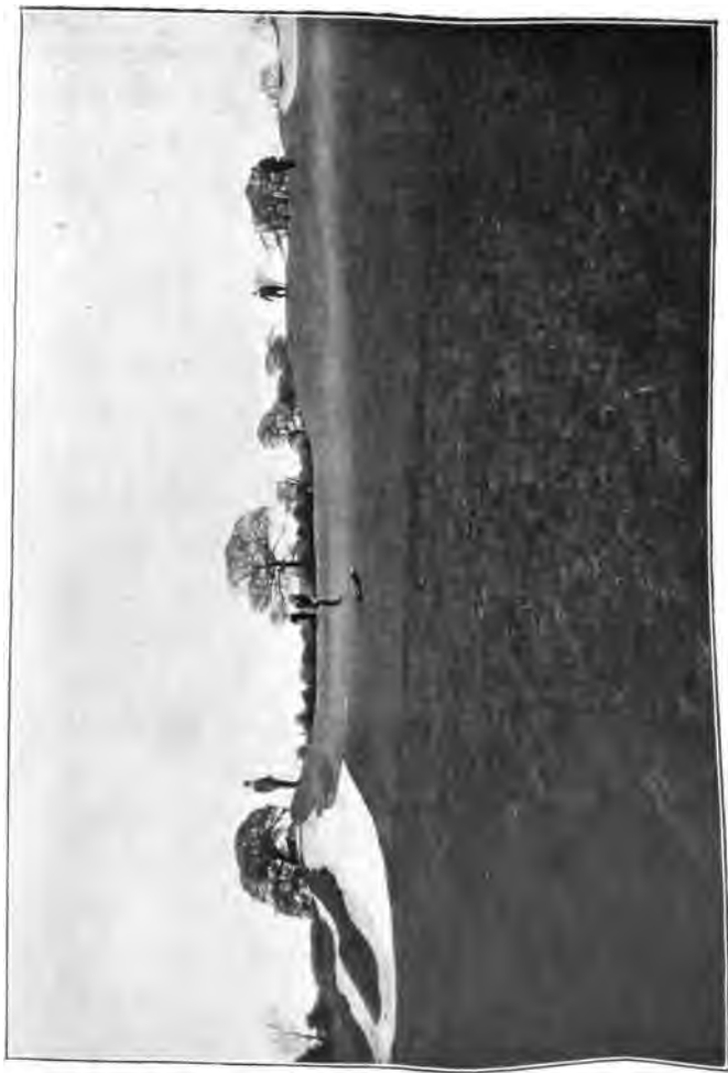
THE SEVENTENTH GREEN AT HARROGATE: APPROXIMATE COST £180: an entirely artificial plateau green constructed on flat land. The comparatively heavy cost is due to the character of the subsoil—heavy clay.
