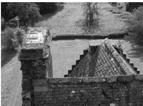
This shows a tree growing out of the east chimney head!
