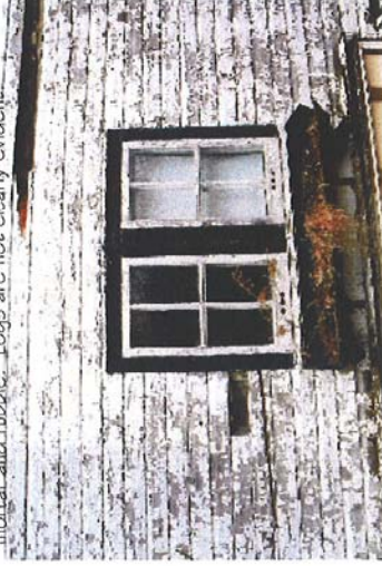
14. Close up of windows and hole in siding where photo 13 was taken.
