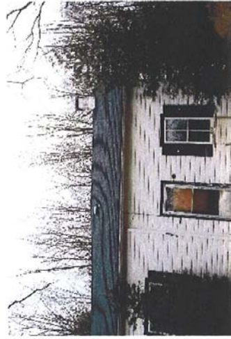
6. The join of the two parts. The east part is set back slightly.
