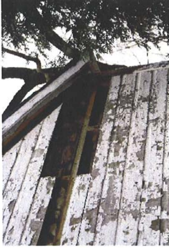
12. Damage at the eaves shows heavy applications of mortar and rubble. Logs are not clearly evident.
