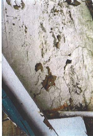
10. Close-up of the cold cellar wall showing a relatively thick layer of plaster over rubble stone. The plaster has a reddish colour indicating a local sand was used.
