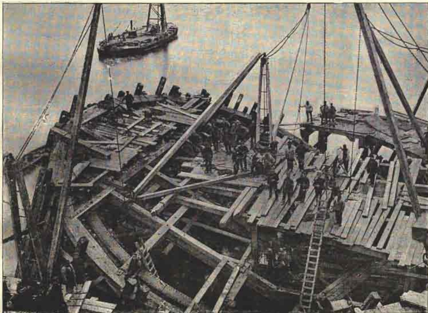
CAISSON FOR QUEENSFERRY NORTH-WEST PIER, CONSTRUCTING TIMBER CASING ROUND THE TILTED CAISSON.
