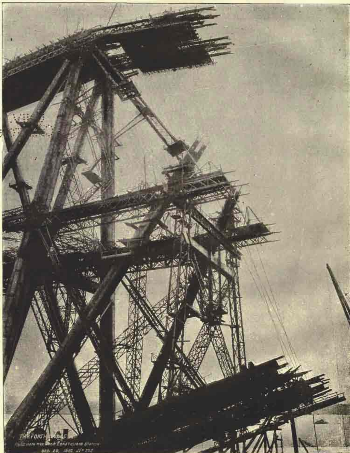
FIVE PIER. FIRST HALF-BAY IN FIXED CANTILEVER, SHOWING LIFTING PLATFORM FOR BUILDING THE LOWER PORTION OF BAY AND TOP MEMBER CRANE WITH PLATFORM SUSPENDED FROM IT.
