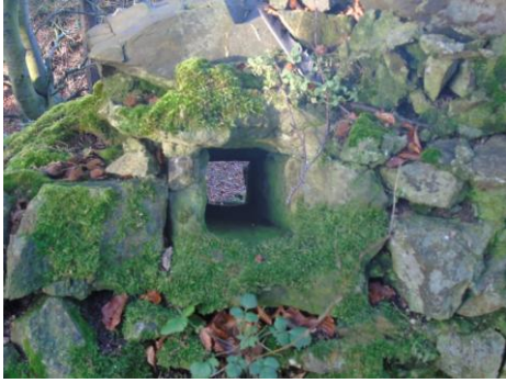
Interesting (spy?) hole in the north wall adjacent to the former gateway. (S. Bruce).
