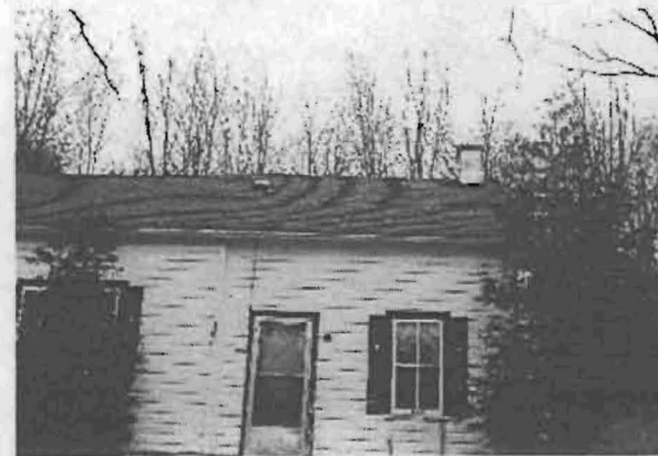
6. The join of the two parts. The east part is set back slightly.
