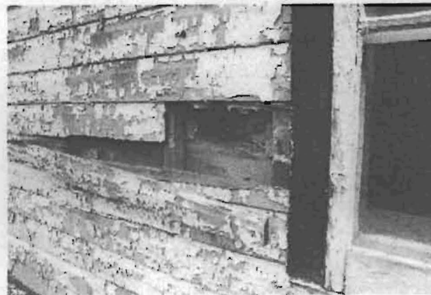
13. The sawn log construction is clearly visible where the siding has been broken. The strapping is old wood indicating that the logs may have had siding added at an early date.
