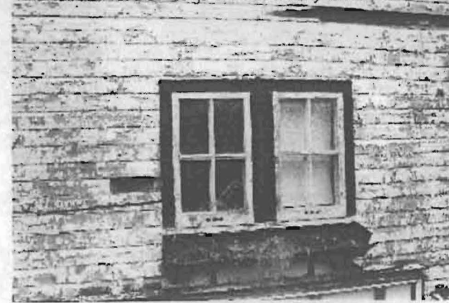
14. Close up of windows and hole in siding where photo 13 was taken.
