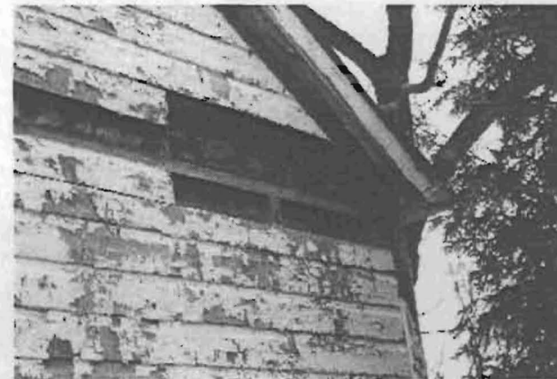
12. Damage at the eaves shows heavy applications of mortar and rubble. Logs are not clearly evident.
