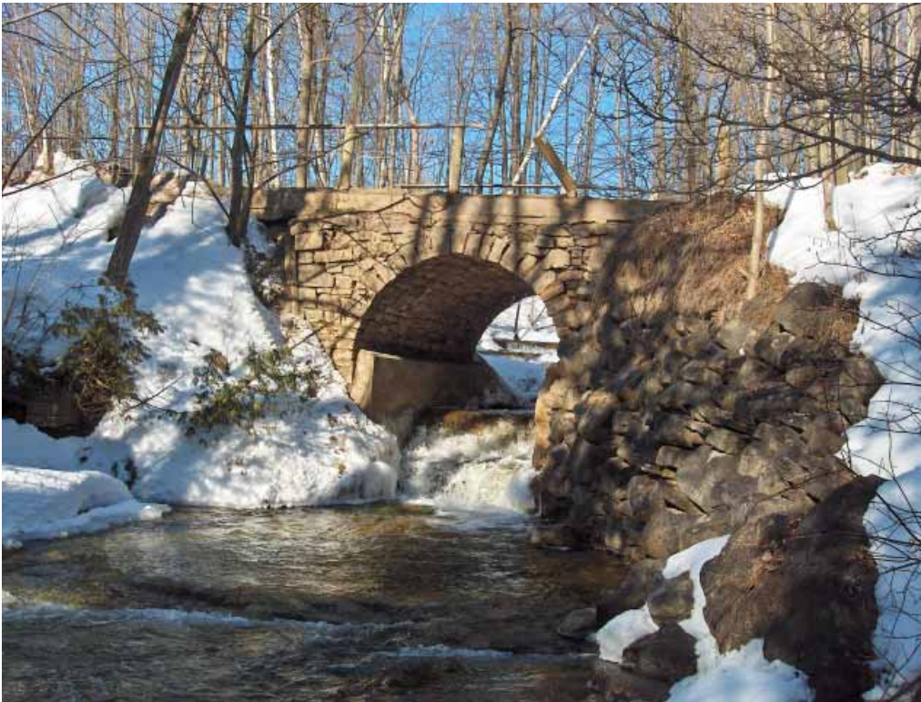
5/06 Silver Creek Bridge (sandstone bedded in lime mortar, single vault) Note modern concrete abutments added to reinforce base of arch, and wooden railing installed on concrete cap laid over masonry. © T.Murison 2008
