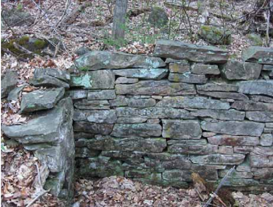
4.16 N.E. corner of stone foundation for mill wheel. Upstream end wall at left.
