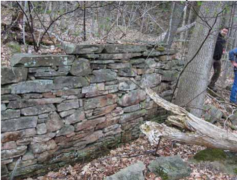
4.17 Portion of earth embanked wall which supported bearing blocks for millwheel. Large (20") hardwood tree has grown up on the debris and stone which has filled the trench. Rob Kier (black jacket in background) a resident of the house, found these walls in 1961.
