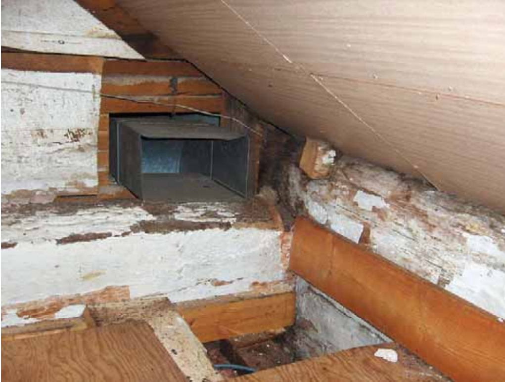
1.42 Interior of McClure/McKay Log House, at top plate. Notice whitewash on logs and interior of gable frame wall. (Pine board on the right side and plywood flooring are modern). The whitewash flakes off in thick chips with visible layers indicating several applications of the mixture, applied over many years of use. © T.Murison 2008
