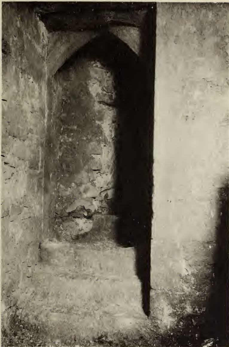
(FIG. 11) VIEW OF DOORWAY FROM ENTRANCE HALL TO INTERIOR OF TOWER, SHOWING LATER ADDITION TO THICKNESS OF WALL
