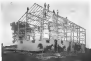
Steel framework was erected for new county government. Work started soon to erect floor-to-ceiling steel wall panels. In photo shown at left, work is shown by more than 100 laborers in early fall of 1939.
